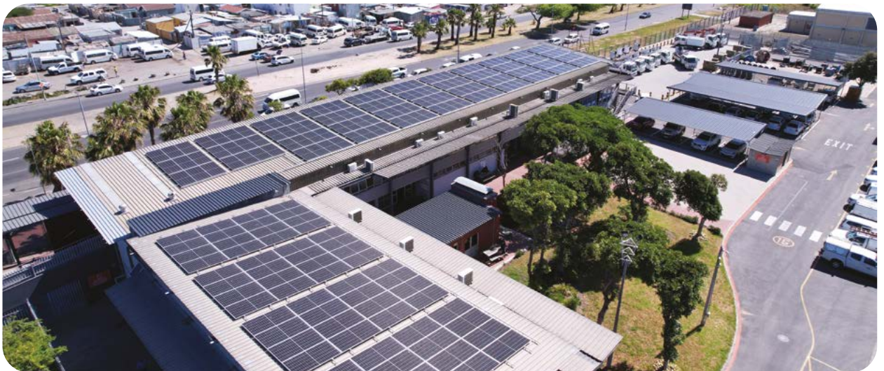
An active programme is in place to help enable the uptake of renewable energy in City buildings.
